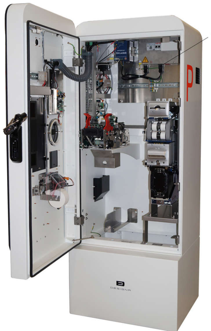
Fig. 40: Measuring point for measuring the fault loop impedance
