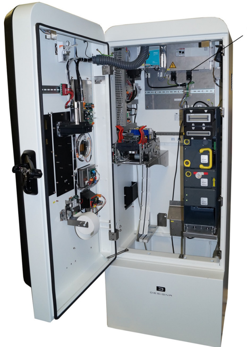
Fig. 34: Measuring point for measuring the fault loop impedance
