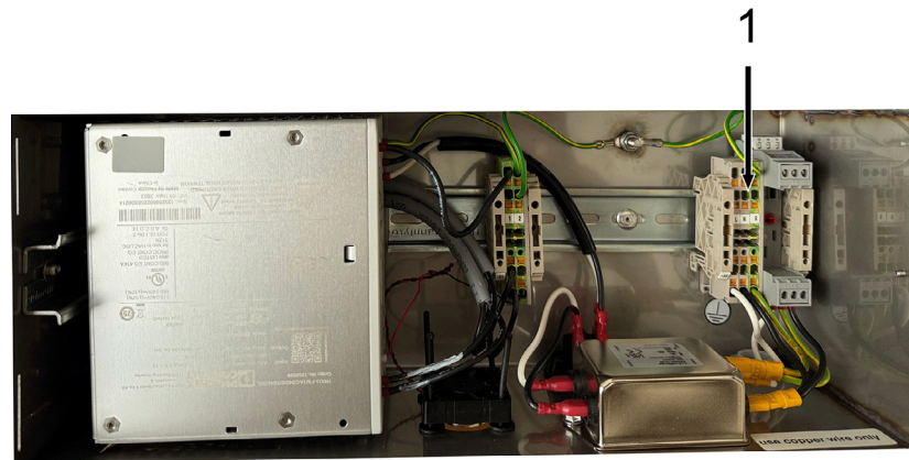
Fig. 27: Measuring point for measuring the fault loop impedance
